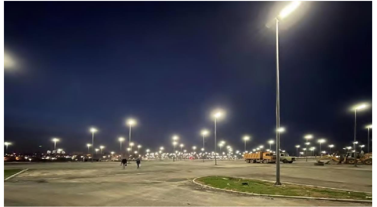
SSL-310 10M 2000PCS Parking lot and road lighting for Oran Stadium project
